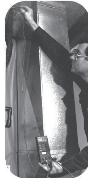
FIGURE 41 TEMPERATURE RISE MEASUREMENT
