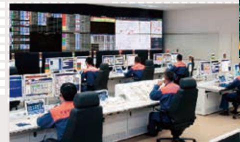
Fireproofing command center
